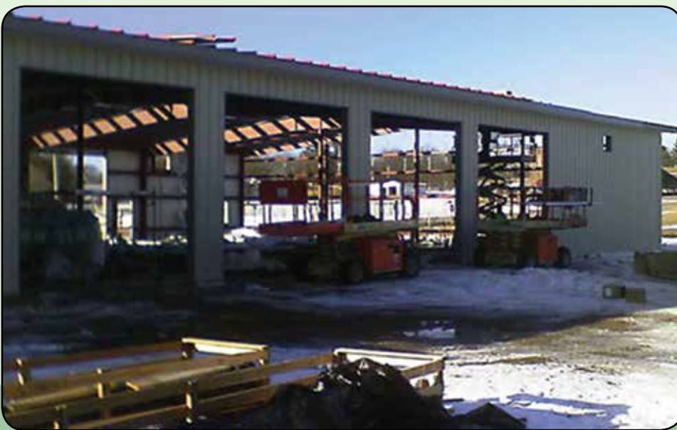
A grant from the SMSC funded construction of a 12,000 square foot fire and ambulance building in the community of Naytahwaush.
